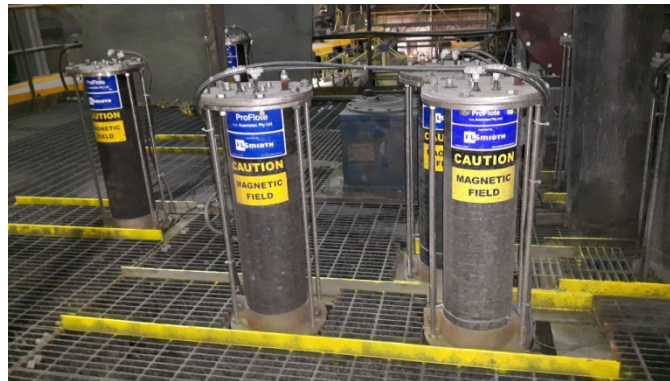
Figure 3 – Magnetic tubes on top of the Cu conditioning tanks
