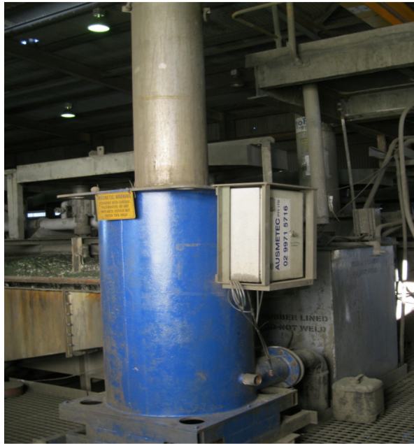
Figure 3 – ProFlote magnetic conditioning installation in the copper circuit
