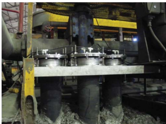
FIG 4 - Magnetic conditioning installations in the retreat bank.
